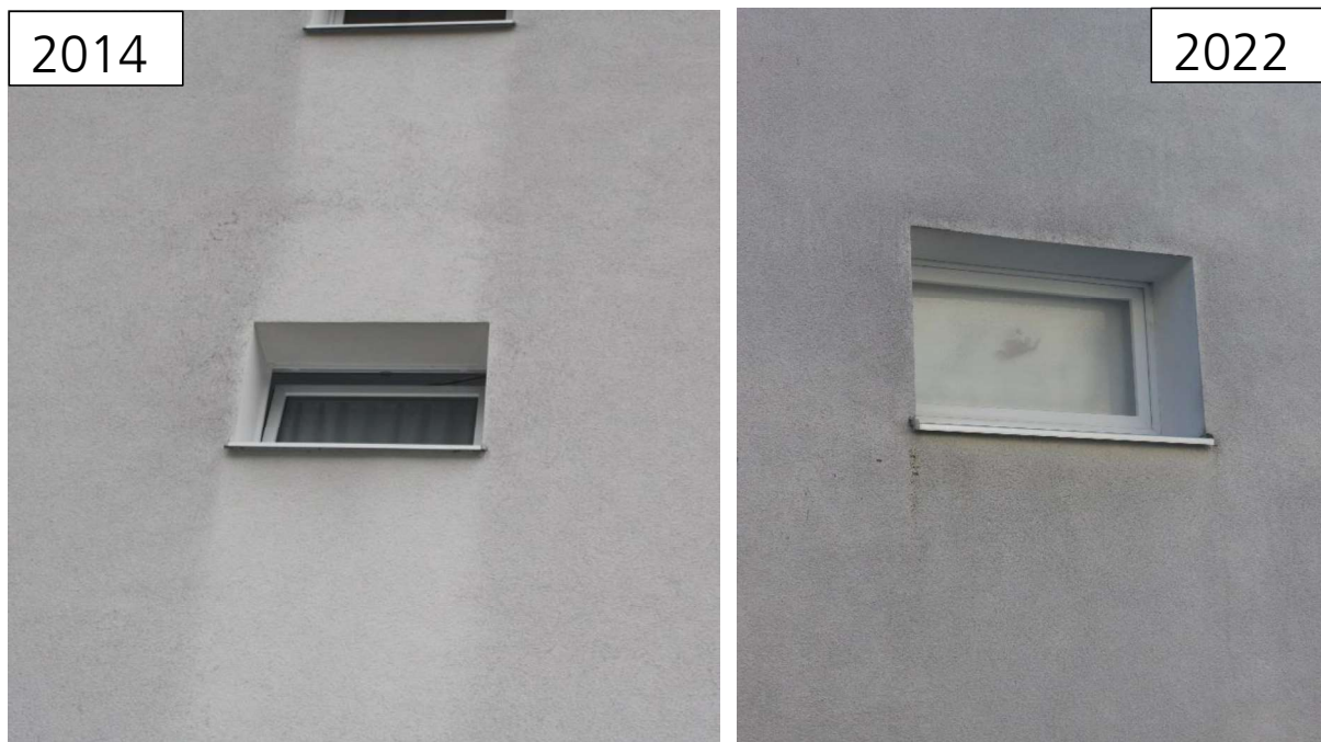
Figure 29: View of the west façade of object 31; in 2014, noticeable color differences could be seen between the area underneath the windows and the undisturbed façade; in 2022 an even graying is visible.
