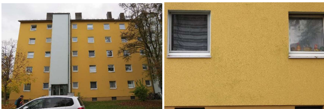
Figure 49: View of the north façade of house number 85, including a close-up of the lower façade surface with algae growth.
