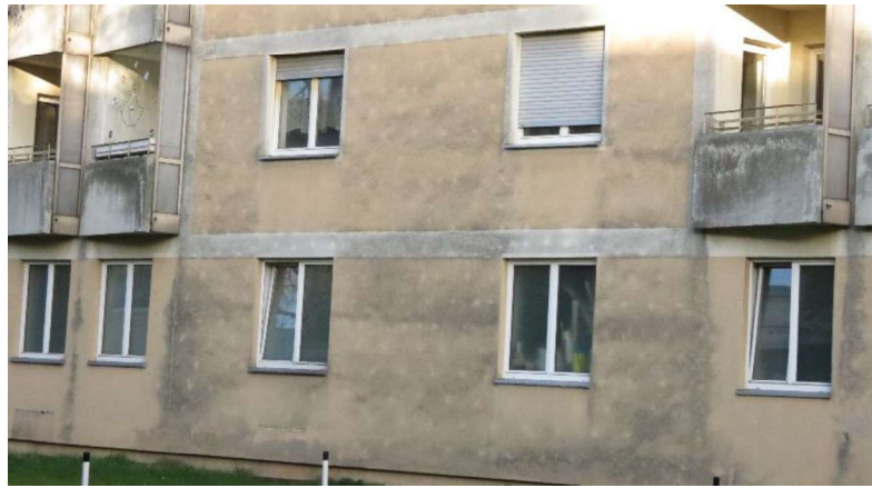
Figure 6: View of the facade of object 16. With noticeable appearance of the dowels on the first and second floor.
