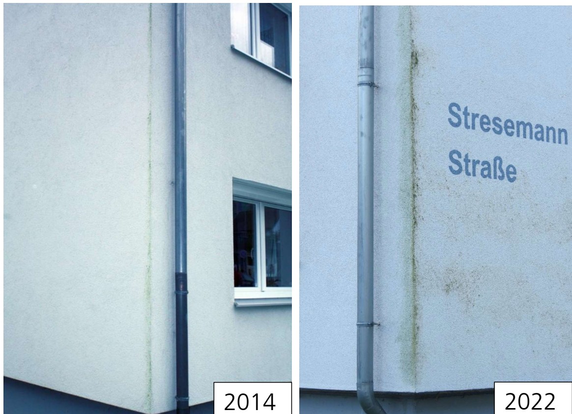
Figure 31: View of the south-west corner of the building in 2014 (left) of object 30 and the north-west corner of the building in 2022 (right) with algae growth on the edge of the building.
