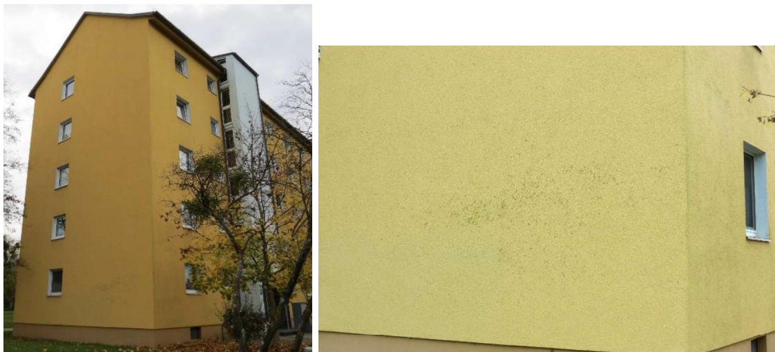
Figure 48: View of the east façade of house number 85, including a close-up of the lower north-east façade surface with algae growth.
