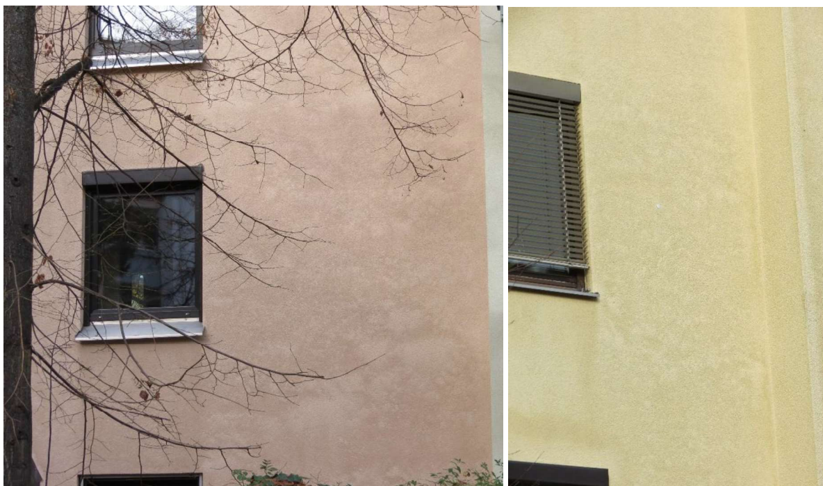
Figure 11: View of the east façade (left) and south-east façade (right) on object 95 with noticeable splotch formation but no crack formation.
