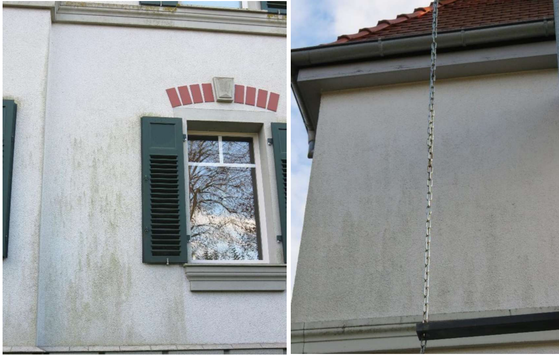
Figure 43: Close-up of the NW façade (left) and SW façade (right) with noticeable green- ing.
