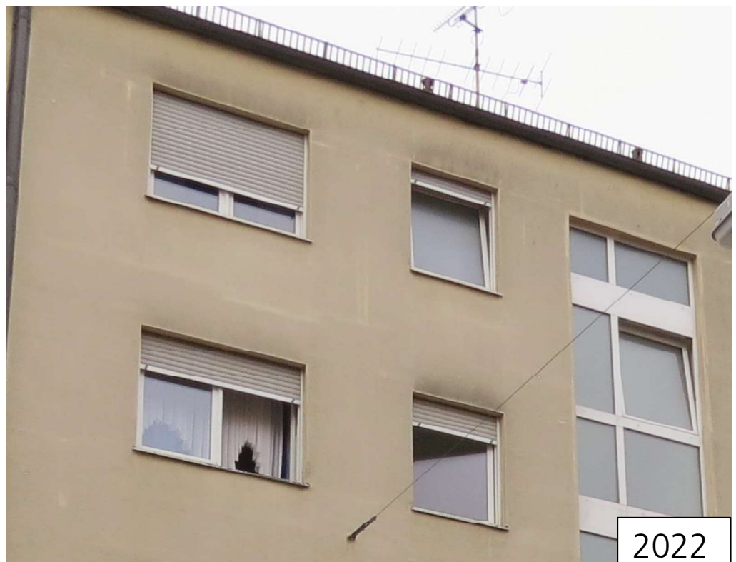
Figure 14: View of the top north facade in 2014 (top) and 2022 (bottom) of object 51 on which noticeable condensation trails and light areas along the panel joints of the ETIC system are clearly visible.
