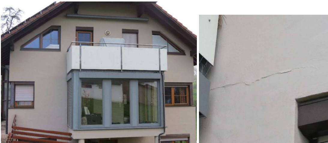
Figure 54: South view of the façade (left) of object 10. Crack formation visible at the upper connection of the conservatory (right).
