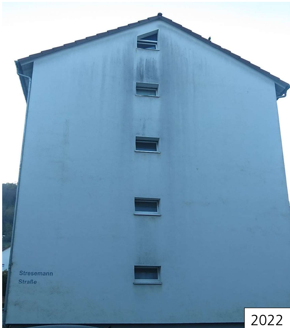
Figure 32: View of the west façade (2022) of object 30 with noticeable condensation trails and the beginnings of algae growth.
